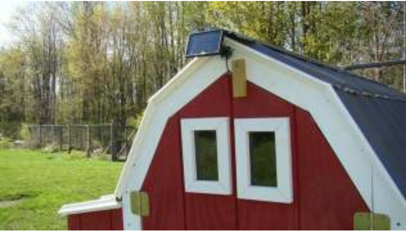
Solar panel faces south
